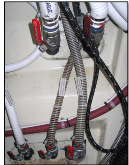
Plumbing and seacocks clearly labeled
