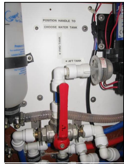
Fresh water distribution system.
